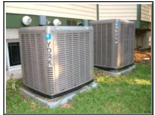
This home has two separate central air conditioning systems. One zone is the main floor, while the smaller unit cools the second floor. PHOTO CREDIT: Tim Carter
