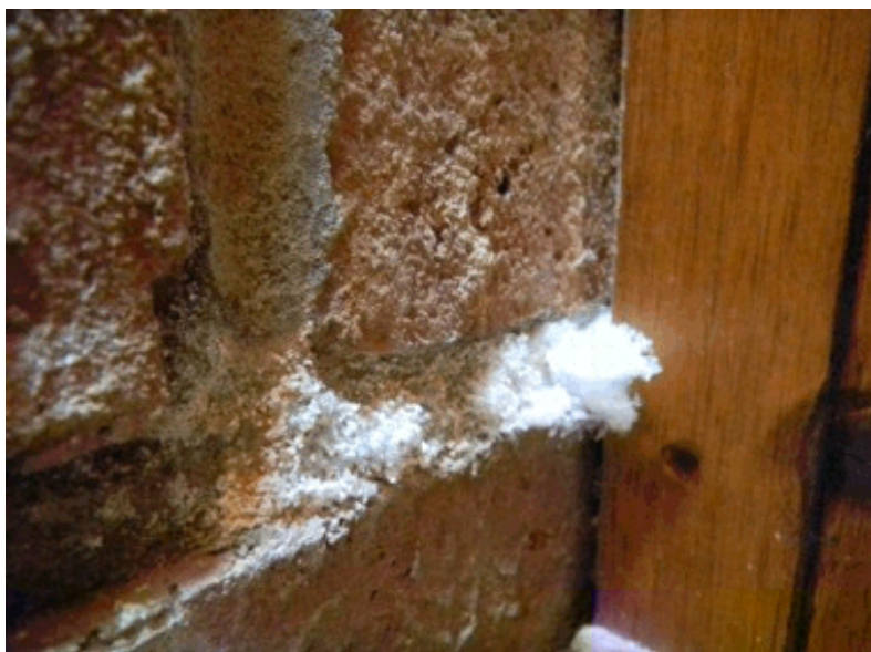
Efflorescence growing in the mortar of a brick fireplace.
