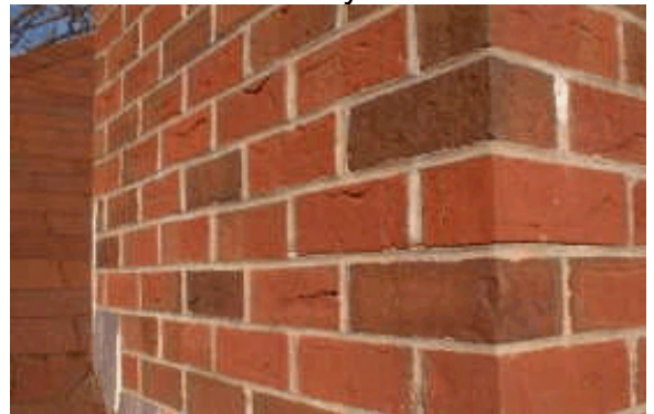
The crack travels the entire length of the horizontal bed joint.
