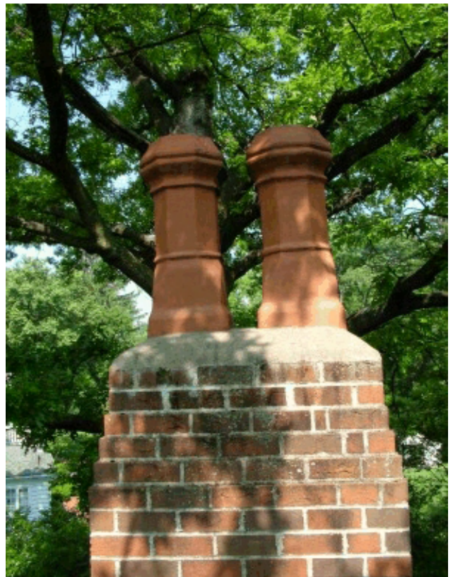
This cement chimney cap is like most. It is lacking an overhang, and it does not have a flashing beneath the cement mortar. PHOTO CREDIT: Tim Carter
