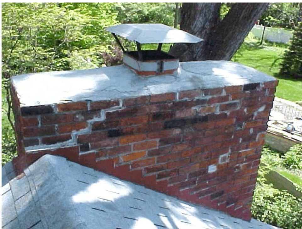
The color of the grains of sand makes a huge difference in mortar color once the actual cement paste wears away. PHOTO CREDIT: Clay Lamb
