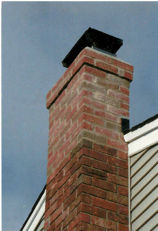
The color of the brick and mortar don't match in this chimney repair. This will be noticeable from the ground. PHOTO CREDIT: Clay Lamb
